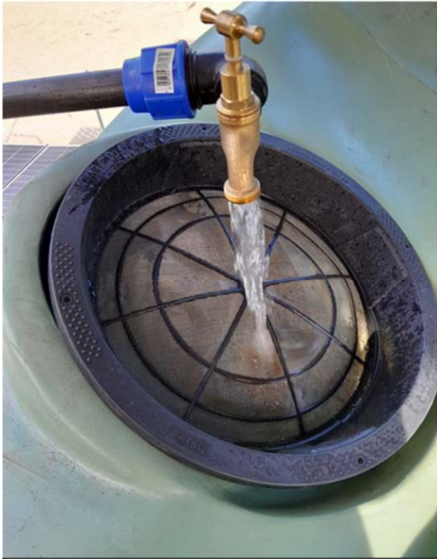
Water pumped by solar into storage tank
