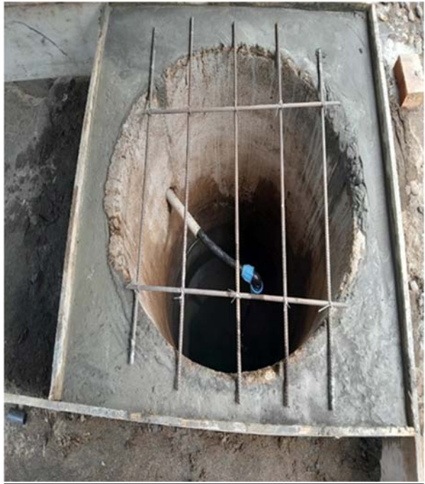
Well built in 1964 - rejuvenated – reservoir
